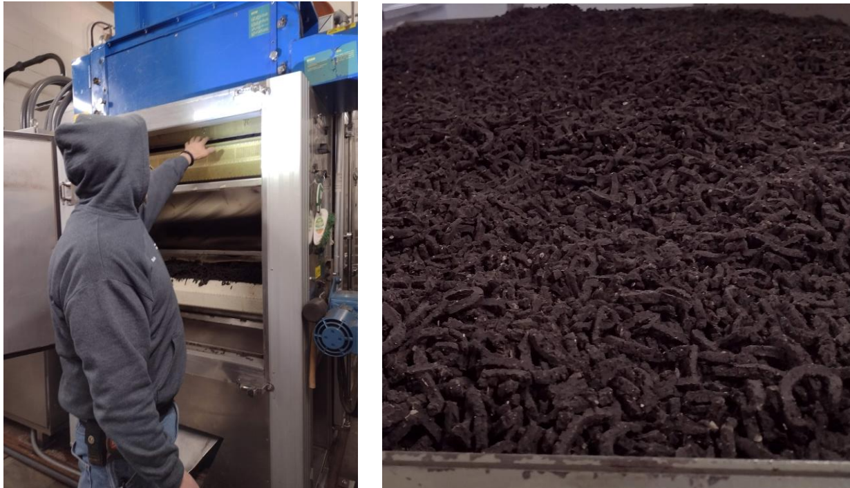
Figure 5. On-site photos at the Bellows Falls wastewater treatment facility. Left: Sludge dryer with panel open, showing conveyer system. Right: Dried Class A final biosolid product. Source: Efficiency Vermont.
