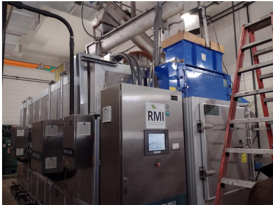
Figure 3. Shincci heat pump sludge dryer installed in Bellows Falls, VT. Source: Efficiency Vermont.
